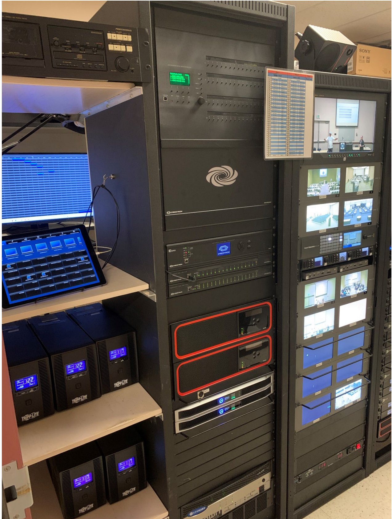
AV Room with Amp Rack and the Biamp and Crestron systems
