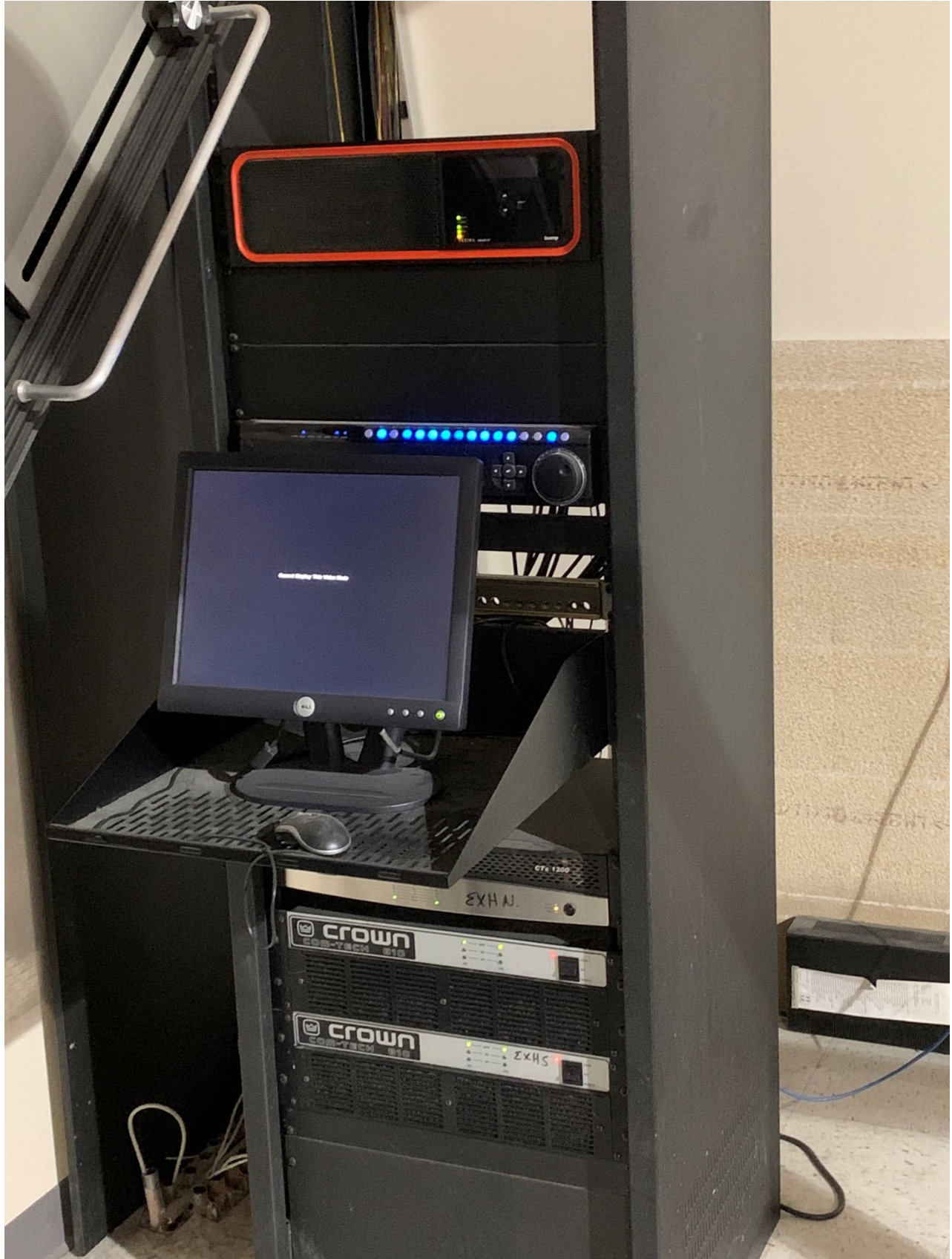
Amp Rack in Sound and Light Booth.
