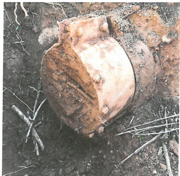
Photo D.1-45 – Northern Chimney Drain Outlet location: Looking northeast. Outlet was found to be full of sediment.
