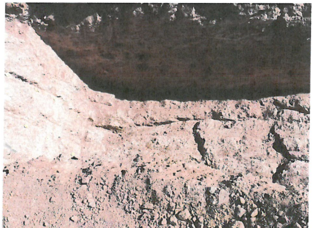
Photo D.2-A3-12 – T-13 location: Looking northeast into trench at the two cracks located in the wall of the middle bench and their continuation further downstream in the floor of the middle bench.
