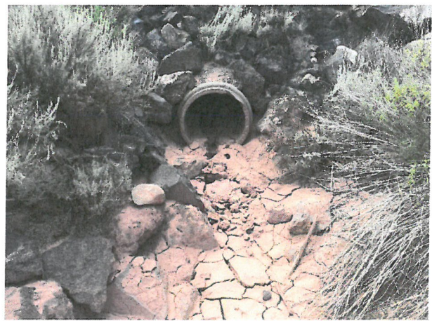
Photo D.1-39 – Principal Outlet location: Looking towards dam along principal outlet prior to any excavation.
