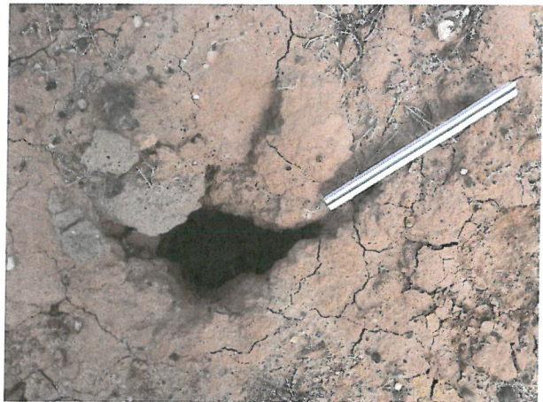
Photo D.2-A3-4 – T-8 location: Looking overlooking H-11 prior to exploration. Remnants of grout from previous maintenance attempts can be observed at the surface.
