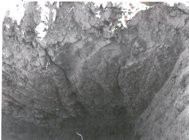
Photo D.2-A5-3 – T-14 location: Looking northeast down into trench at the northeast wall. The chimney drain can be seen in the middle of the photo.
