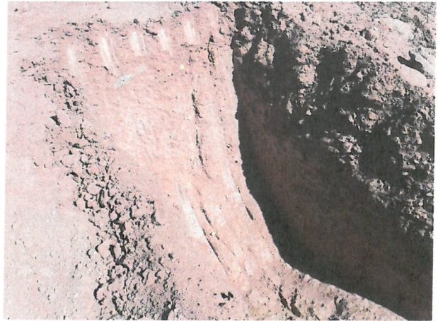
Photo D.2-A3-11 – T-13 location: Looking northwest into trench at the crack located in the upper northwest wall.
