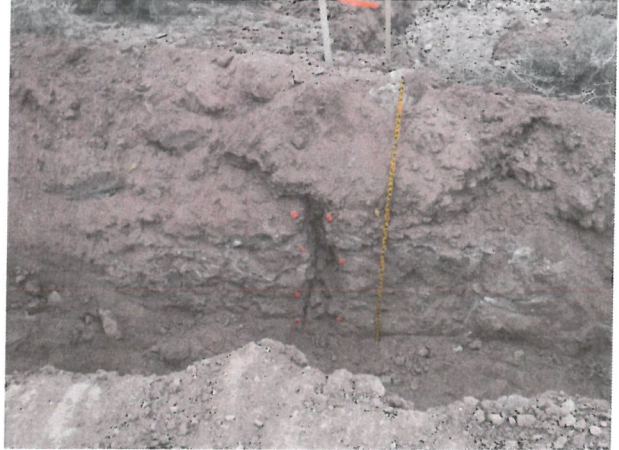
Photo D.2-A2-8 – T-12 location: Looking northwest into trench at continuation of crack through northwest wall.
