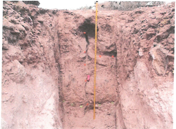
Photo D.2-A4-8 – T-11 location: Looking northwest. A transverse crack can be observed in the northwest wall and a 3 inch hole intersecting the crack and running longitudinally in a northeasterly direction along the dam.
