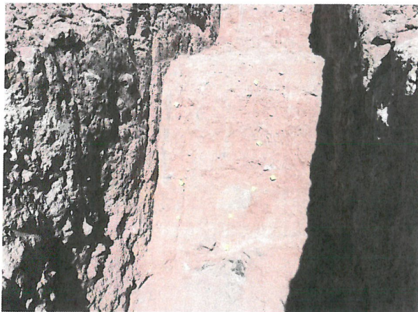
Photo D.2-A3-13 – T-13 location: Looking northwest along T-13 showing the continuation of two cracks into the lower wall, and finally terminating at the underlying basalt formation
