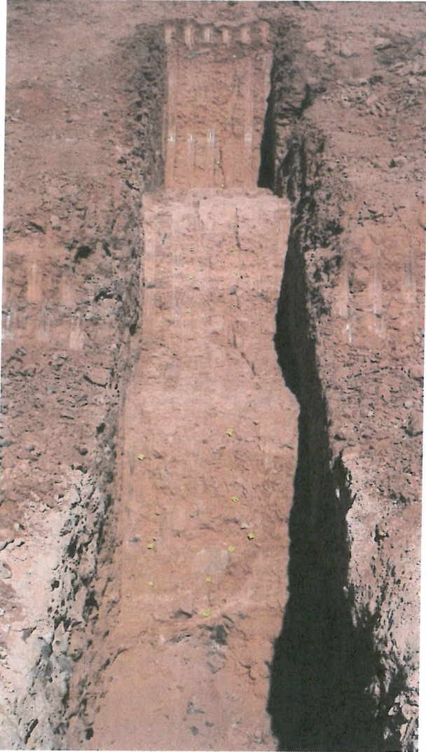
Photo D.2-A3-14 – T-13 location: Looking northwest along T-13 showing the continuation of two cracks into the lower walls, and finally terminating at the underlying basalt formation
