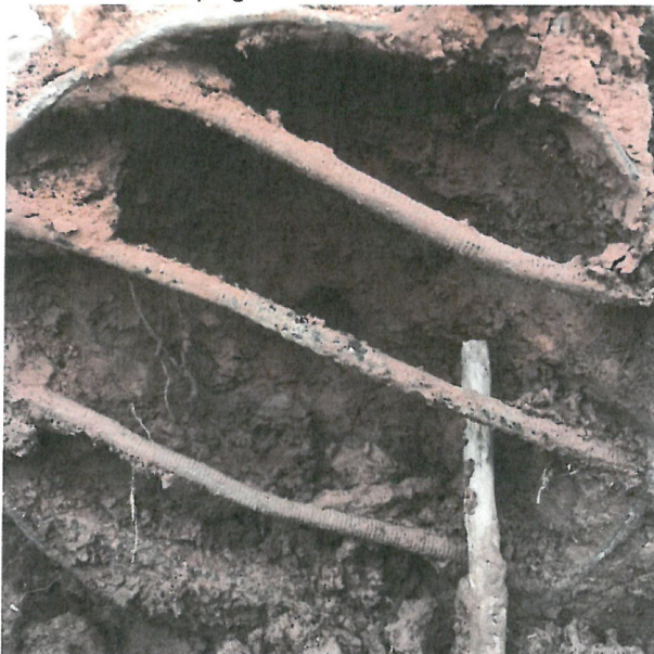
Photo D.1-44 – Southern Chimney Drain Outlet location: Sediment within outlet extends more than 6" into pipe.
