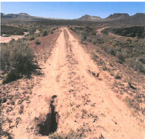
Photograph 7: Sinkholes H-6 & H-5 up to 18 inches wide along crest of embankment; view to north.
