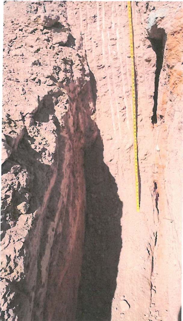
Photo D.2-A3-9 – T-8 location: Looking northwest after excavation was completed. An open crack can be observed in the northwest wall below grout cap, and in the floor of trench.
