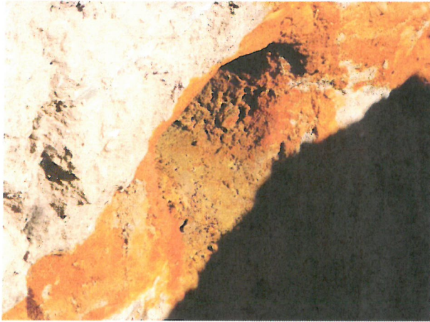
Photo D.2-A2-3 – T-5 location: Looking northwest into trench at staining around 10-inch hole in chimney drain material located on the northwest wall.
