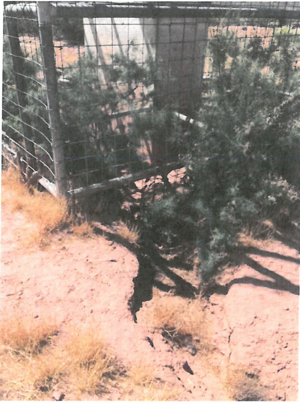
Photo D.1-36 Erosion at north corner of drainage structure, vegetation in cage.
