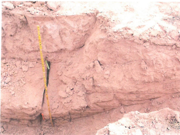
Photo D.2-A4-5 – T-10 location: Looking southeast into trench. A transverse crack can be observed in the southeast wall.
