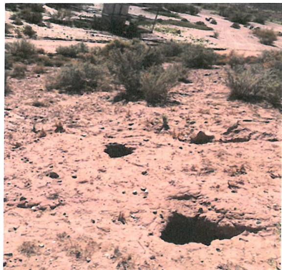
Photograph 8: Several sinkholes 13 to 22 inches in diameter along upstream slope (such as H-43 –H-45).
