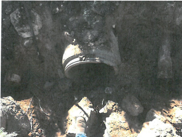
Photo D.1-42 – Principal Outlet location: Looking towards dam down at outlet after exposing chimney drain outlet pipes. One chimney drain outlet pipe is located on each side of the principal outlet pipe; Found at 24" below slope grade.
