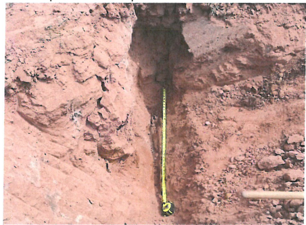
Photo D.2-A1-10 – T-3 location: Looking northeast toward T-4 along longitudinal crack in floor and northeast wall.
