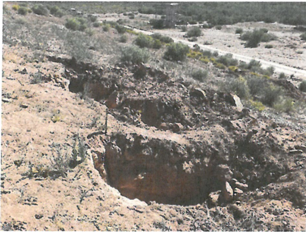
Photo D.2-A1-7 - T-2 location: Looking northeast along general northeasterly direction of the longitudinal crack. Longitudinal crack is located in northeast wall of T-2 directly below wood stake (center left).
