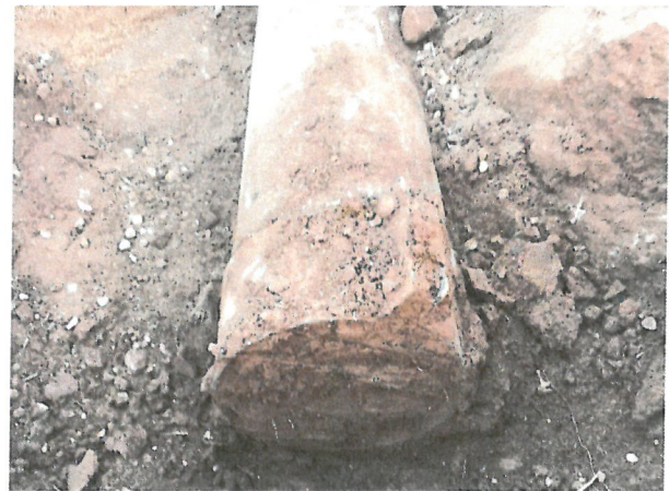
Photo D.1-43 – Southern Chimney Drain Outlet location: Looking towards dam. Outlet was found to be full of sediment.
