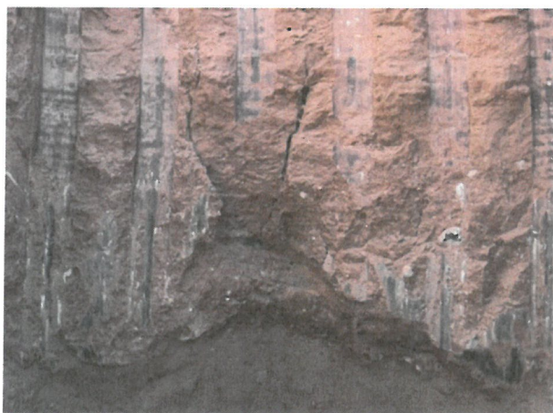
Photo D.2-A5-5 – T-14 close up of crack in southeast wall.
