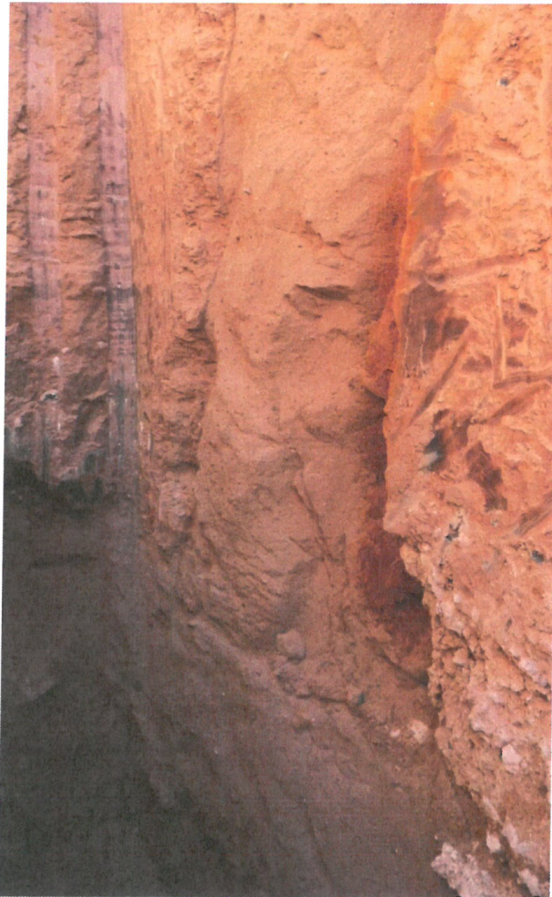
Photo D.2-A5-9 – T-8 location: Looking at the staining in the southwest wall along the chimney drain embankment interaction from the presoaking of holes H-34 & H-35.
