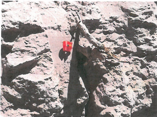
Photo D.2-A2-11 – T-15 location: Looking southeast at the primary transverse crack in the lower wall of T-15. Roots can be observed within the primary crack.
