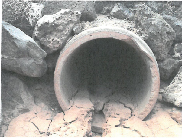
Photo D.1-40 – Principal Outlet location: Looking towards dam along outlet. Sedimentation is apparent in the principal outlet pipe.
