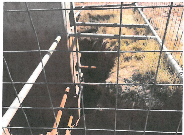
Photo D.1-35 Sediment buildup and erosion at southeast face of drainage structure.
