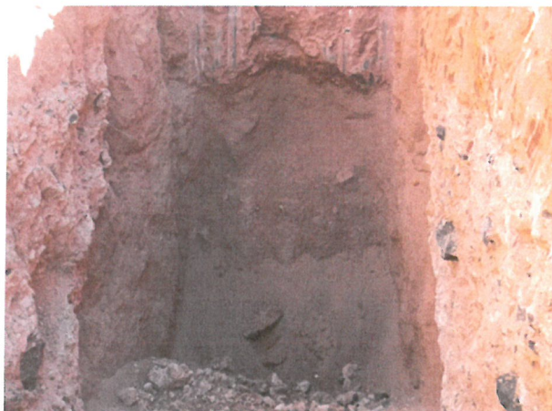
Photo D.2-A5-4 – T-14 location: Looking southeast into embankment. A crack can be observed at the top middle of the photo at the interaction between the embankment material and the chimney drain.
