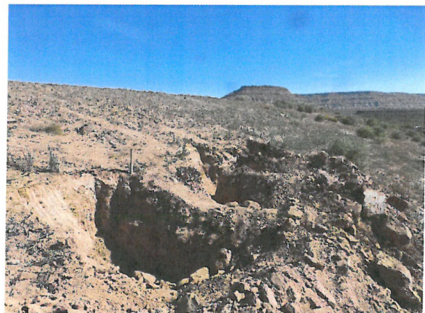
Photo D.2-A1-6 – T-2 location: Longitudinal crack is located in northeast wall of T-2 directly below wood stake (center left).
