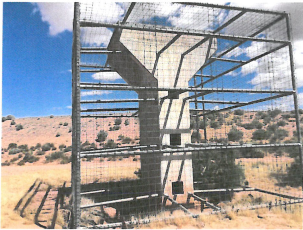
Photo D.1-32 Southeast face of drainage structure, two openings below ground-surface elevation.
