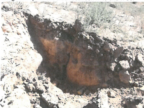
Photo D.2-A1-11 – T-4 location: Looking northeast along the upstream side of the dam showing longitudinal crack in northeast wall.
