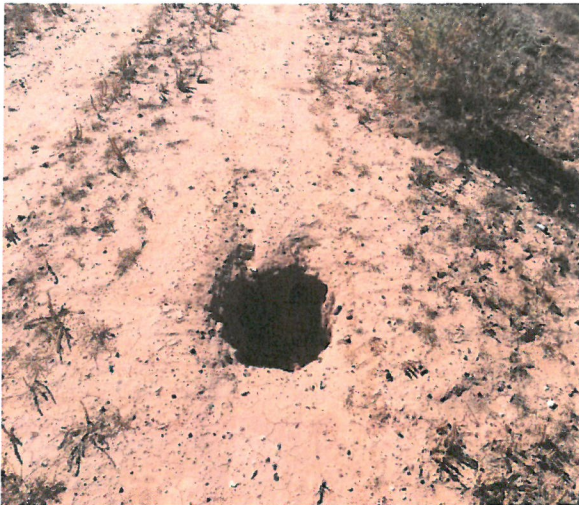
Photograph 5: Sinkhole H-2 about 18 inches in diameter along crest of embankment.
