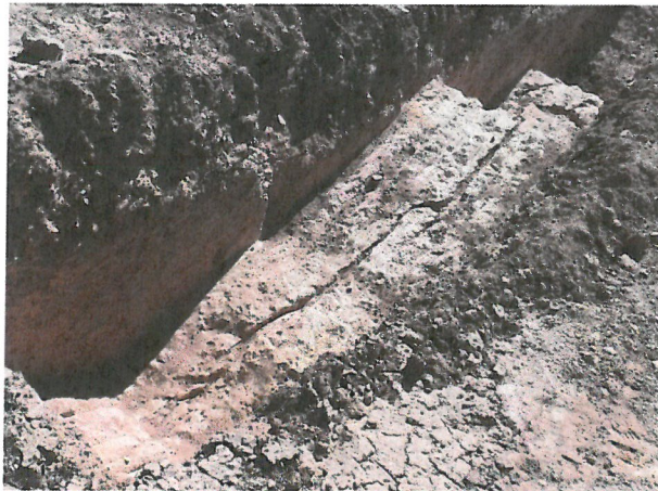
Photo D.2-A3-11 – T-13 location: Looking northeast into trench at the crack located in the floor of the upper bench.
