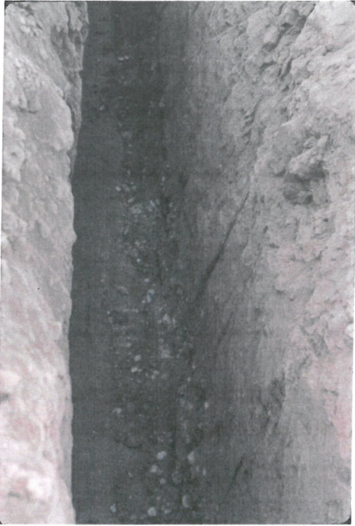
Photograph 3: Exposed transverse cracks.
