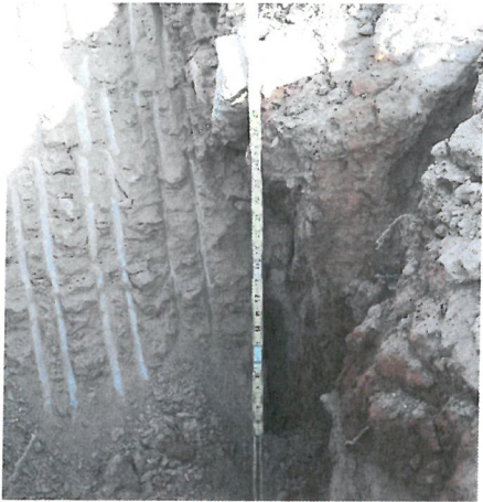
Photo D.2-A3-7 – T-8 location: Looking northwest after 36 inches of excavation at H-11. A grout cap from previous maintenance attempts can be observed to end directly below the surface.
