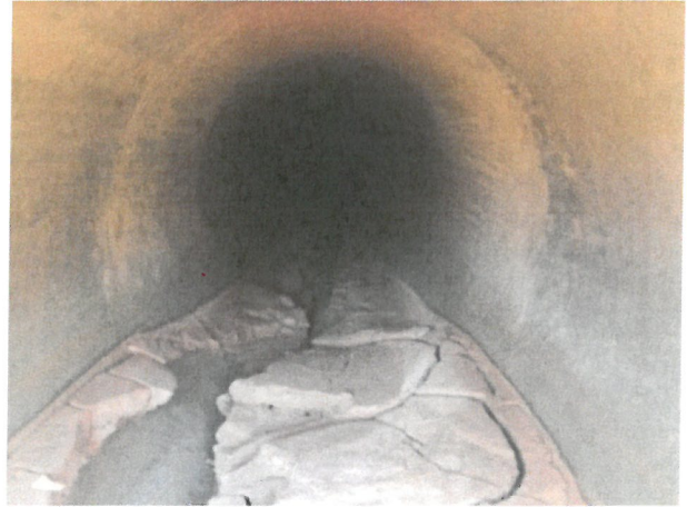
Photo D.1-41 – Principal Outlet location: Looking towards dam into principal outlet. Sedimentation extends back into outlet pipe.
