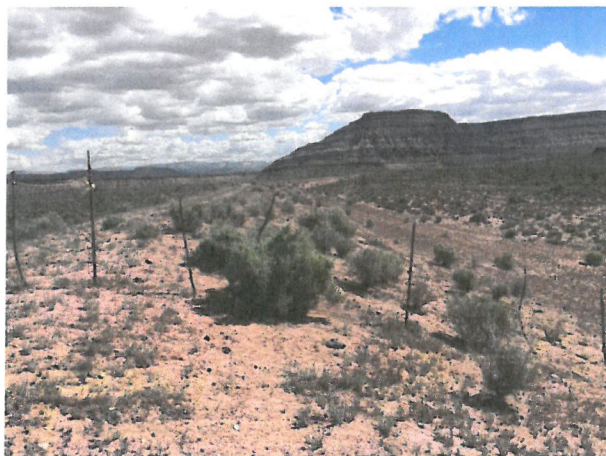
Photo D.1-28 Looking northeast along the downstream slope of the dam, fence crossing dam.
