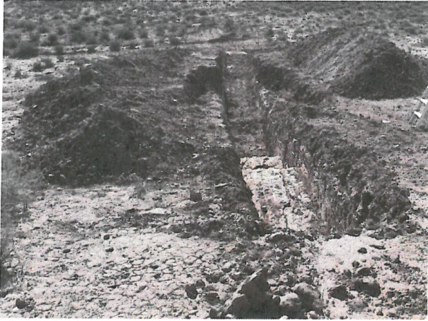
Photo D.2-A3-10 – T-13 location: Looking southeast into the trench from the upstream side of the embankment. Transverse cracking is visible in the floor of the trench.
