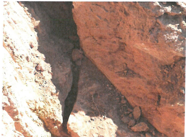
Photo D.2-A1-4 – T-1 location: Looking northeast toward T-2, T-3, and T-4 along longitudinal crack in floor and northeast wall.
