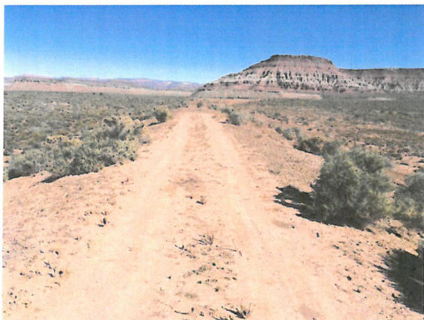
Photo D.1-26 Looking northeast along the center of the dam, knee-high vegetation.
