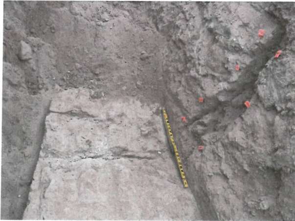
Photo D.2-A2-9 – T-12 location: Looking southwest into trench at continuation of crack in floor through the chimney drain to the left to the downstream embankment to the right. Two separate crack are located in the floor of the trench and appear to converge in the northwest wall.
